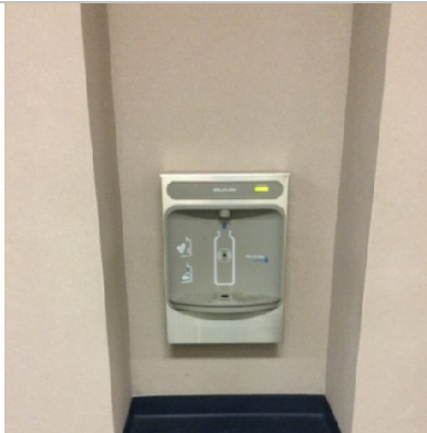
Include an accessible mounted water cooler when space allows
