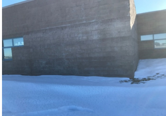
Investigate reason for efflorescence
