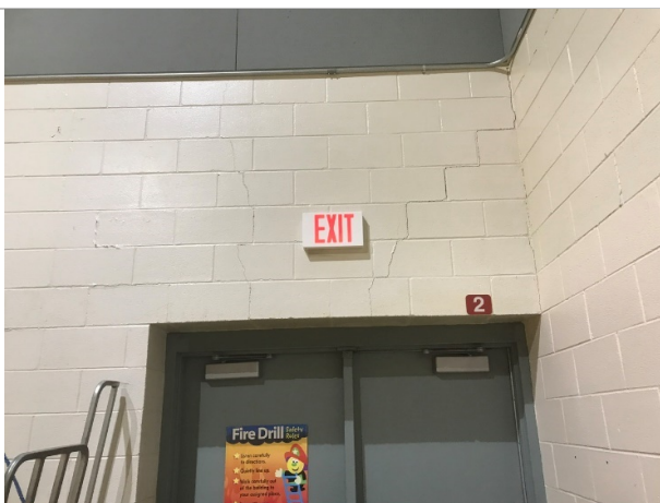
Investigate structural issues
