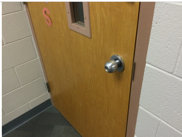
Provide ADA-compliant door hardware
