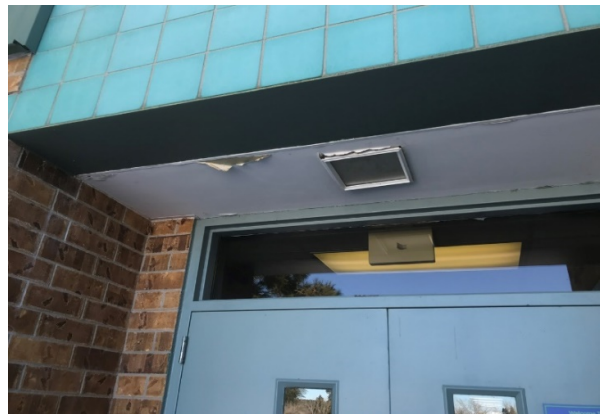
Replace soffit with a more durable material
