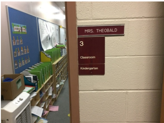
Provide ADA-compliant room signage
