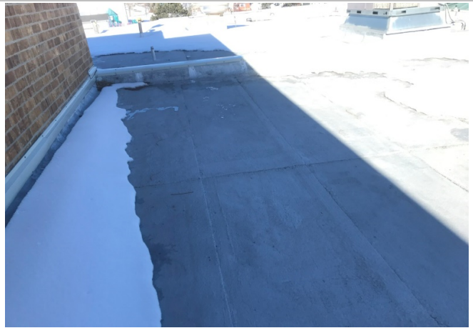
Investigate bubbling at roof
