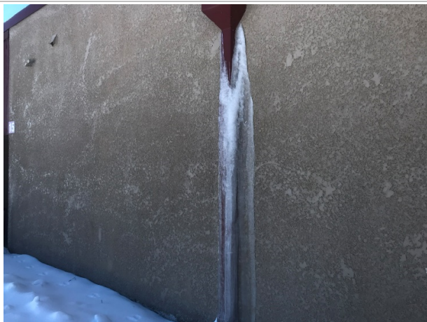
Provide solution for ice buildup at downspouts
