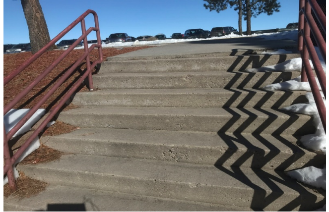
Provide compliant stairs at SW corner
