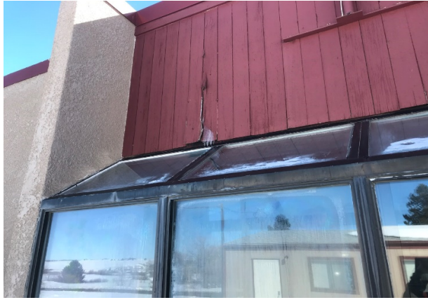
Replace wood fascia with a more durable material
