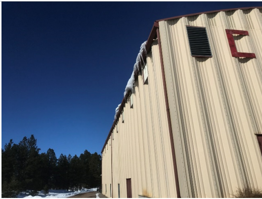
Replace soffit with a more durable material
