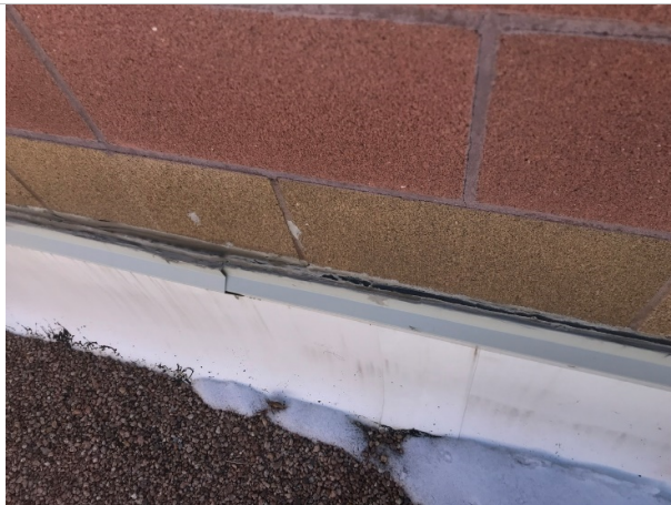
Recaulk between CMU and Flashing on roof
