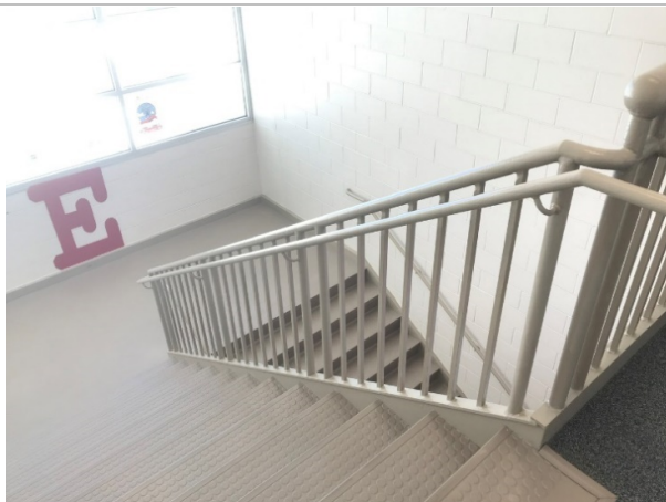
Raise guardrail and handrail height
